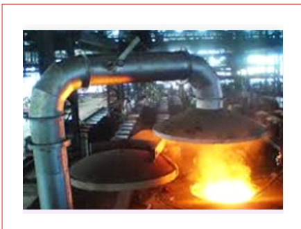
Fume Extraction System
