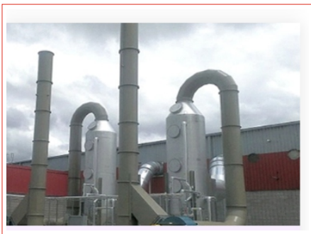
Wet Fume Scrubber
