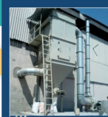
CENTRALIZED DUST COLLECTION SYSTEM
