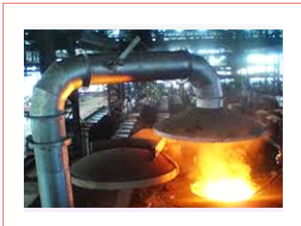
Fume Extraction System
