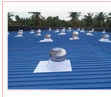
Wind Roof Ventilator
