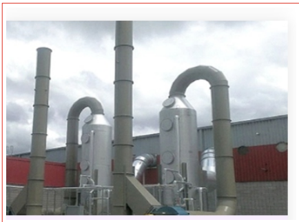
Wet Fume Scrubber
